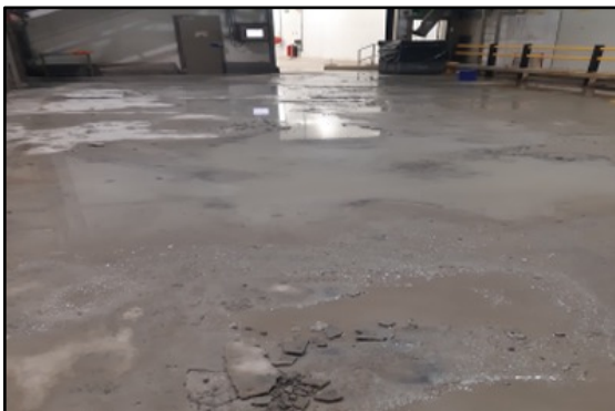
Floor condition with concrete spalling.
